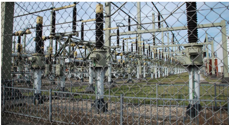
Figuur 16, Schakelstation 150Kv (TenneT)
