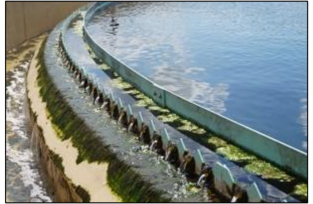
Figure 15, WTP Settling Tank. Retrieved From: http://blogs.edf.org/growingreturns/2015/09/01/why-wastewater-treatment-plants-are-investing-in-farmers/
