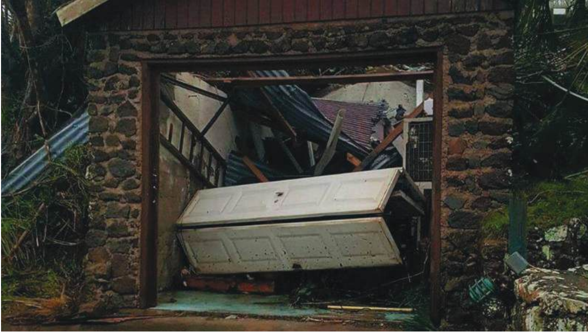
Figure 3.5 A shed with collapsed roof on Saba after hurricane Irma (photo by Aron Hoogendoorn)
