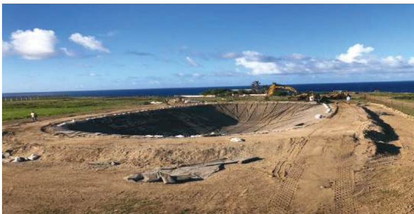
Figure 4.4 Water retention pond under construction near the St. Eustatius solar park. Source: St. Eustatius government
