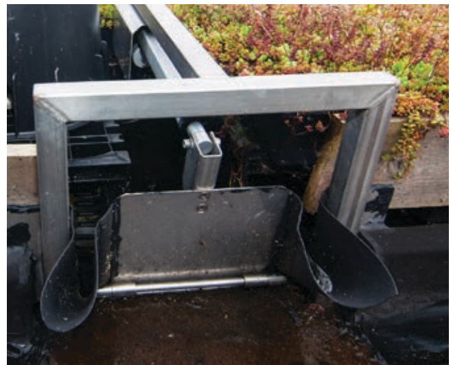
A remotely controlled polder roof system.
